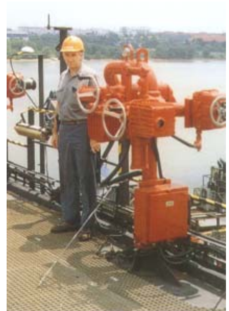
Mr. Geoff Wood, Area HSE Manager, Western Geophysical, during installation / commissioning of WFHC High Volume Remote Control Foam / Water Monitors aboard MV "Western Legend".
